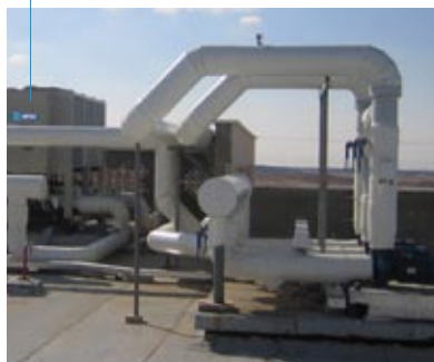
Process cooling application
